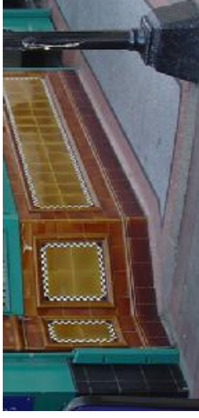
An example of a traditional tiled stall riser at F. Doyles butchers.
