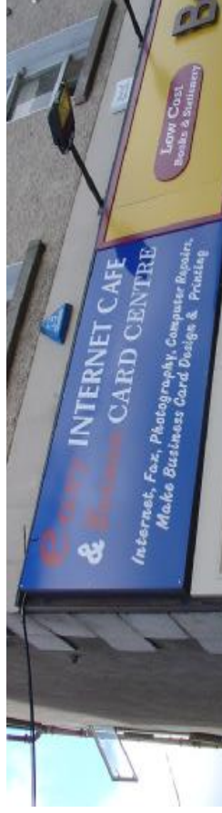
Temporary looking fascias should never be used.
