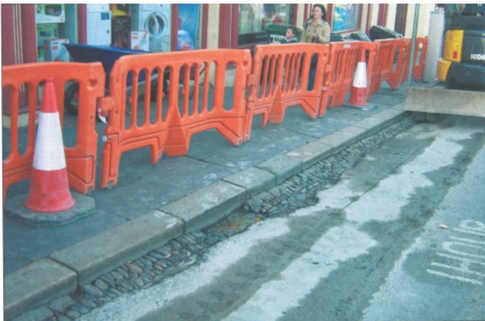
Famine Relief Works, drains on Abbey Street Wicklow Town prior to being covered over by tarmacadam during road surfacing in 2010. Courtesy of John Finlay (2013).
