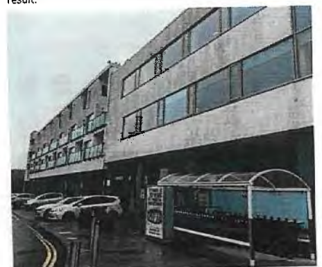
Development at Newtown Square is showing signs of wear, along with the block paved car park which is failing at key junctions due to stress by vehicles.
