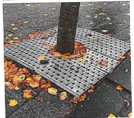
Existing trees along Newtown Square showing signs of tree root egress which is lifting the paving within the canopy diameter of the tree. Some areas of paving have become a trip hazard as a result.
